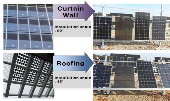
Fig. 8 BIPV system installation in the building
