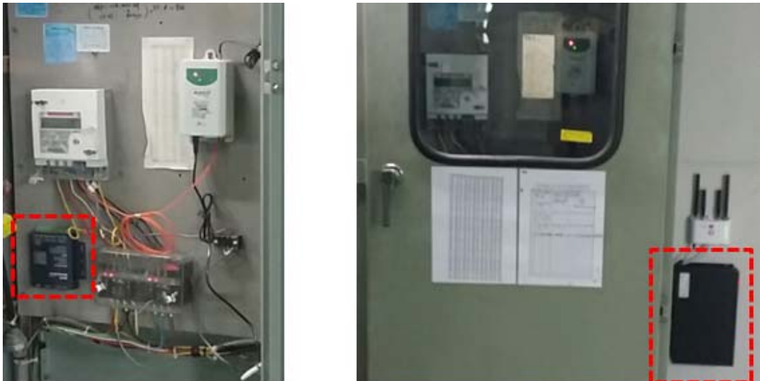
Fig. 3 Smart Box installed at customer site
