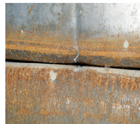
(a) Crack of Z-shaped side plate
