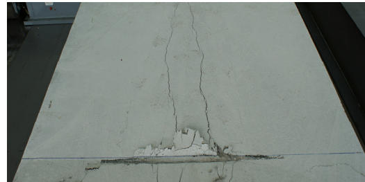
(c) Longitudinal crack of concrete slab
