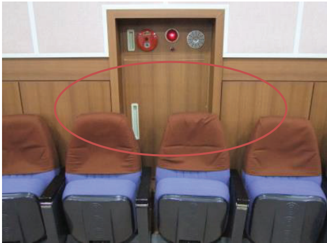
Figure 5. Problems of closed a Fire hydrant
