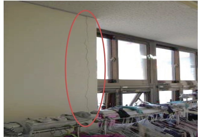
Figure 6. Problems of cracks on walls
