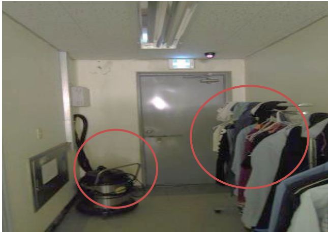
Figure 4. Problems of Church Exit
