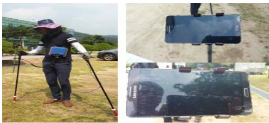
Fig. 19. Defect detection by using a developed DCVG equipment and the monitor.
