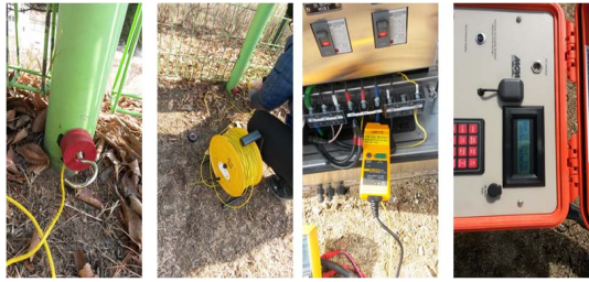
Fig. 15. Installation of an anode and an interrupter for pipeline coating defect detection.
