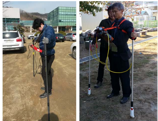
Fig. 12. Pipeline coating defect detection using 2 types of DCVGs.
