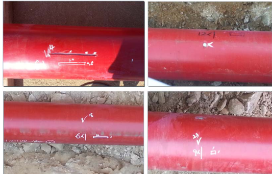
Fig. 8. Artificial coating defect on the pipe installed in the test site.
