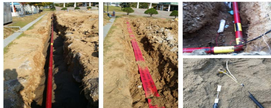
Fig. 9. Installation of pipelines with a magnesium anode and a corrosion coupon in the test site.
