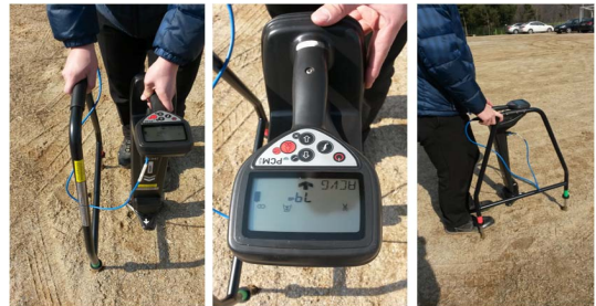
Fig. 11. Pipeline defect detection using ACSVG.
