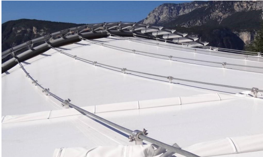
〈Fig. 2〉 Trolley device in the retractable roof Amphitheatre Lavis
