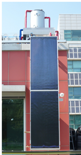
Fig. 4. Natural circulation solar hot water system installation
