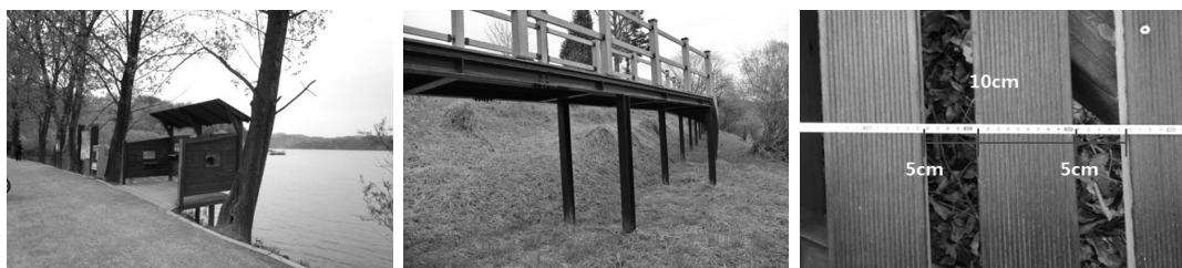
Lack of sheltering at bird observation deck surroundings
