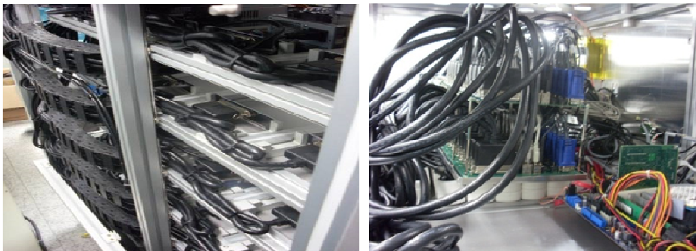
Fig. 1 Cables for DOS system
