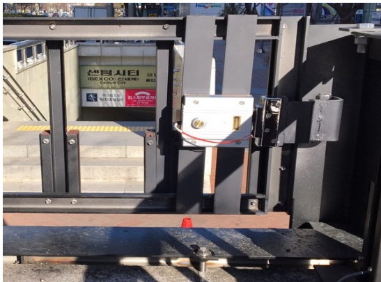
Fig. 2 Door-lock system exposed subway vent
