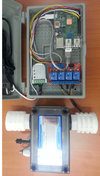
Fig. 9 Control system hardware
