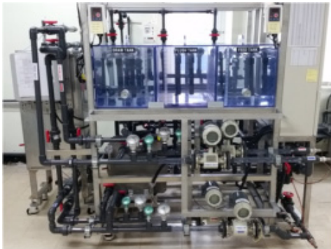
Fig. 2 FO system using six plate-and-frame FO membrane elements
