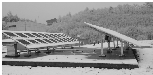
Fig. 1. snow-removal PV & General purpose PV test bed image
