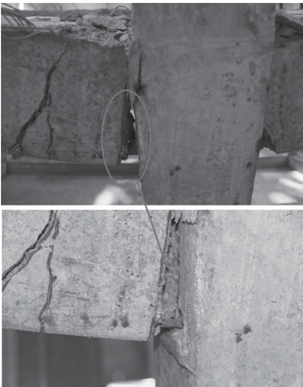
Fig. 10 Rupture of steel bar in A-axis frame beam.
