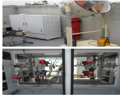
Fig. 1 Test-Bed of Low-pressure Hydrogen Use Facilities
