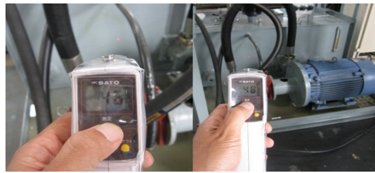
Fig. 13 Temperature measurement of oil tank
