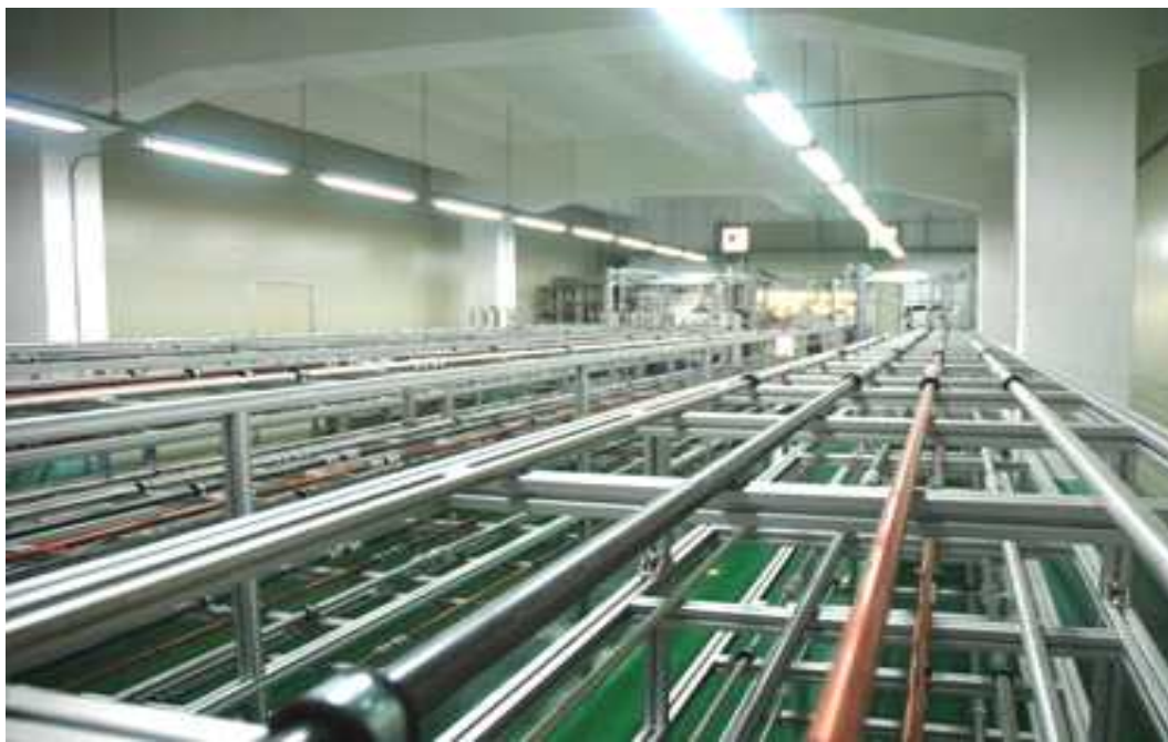
Fig. 3. Test pipes in demo plant consisting of carbon steel, copper, galvanized iron, cast iron.
