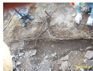
(a) Occurrence of roots penetration to concrete cracks
