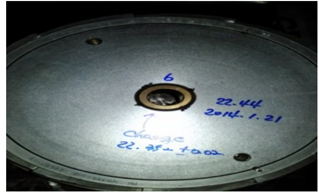
Figure 3. Bushing abrasion status of pump.
