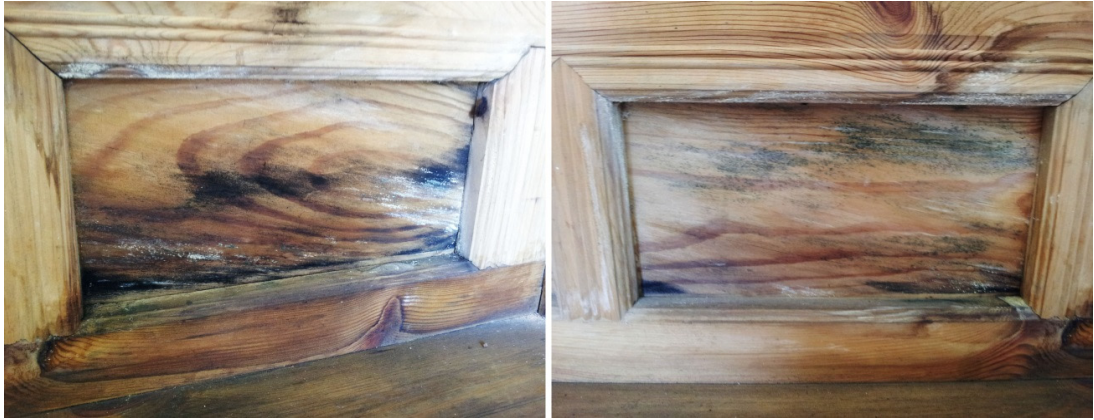
Fig. 3. Severe surface mold damages of the interior of Cheonseokjeong.
