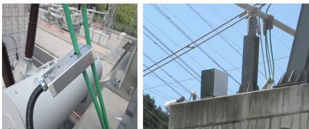
Fig. 5. Protective enclosure and sensor case at SINPOCHEON Substation.
