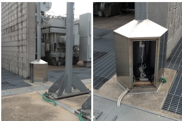
Fig. 2. Protective enclosure and sensor at SINGAPYEONG Substation.
