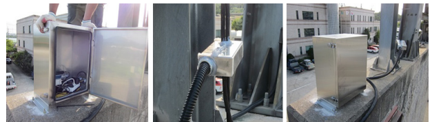
Fig. 3. Protective enclosure and sensor case at MIGEUM Substation.
