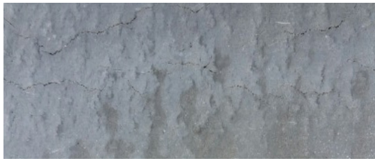
Photo 4. Micro cracks after steam curing (OPC20FA80)
