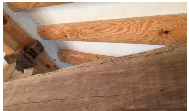
Fig.2 Termites Damages in Wood Beam of Old Wooden Heritage (Gye-jeong of Dokrak-dang)
