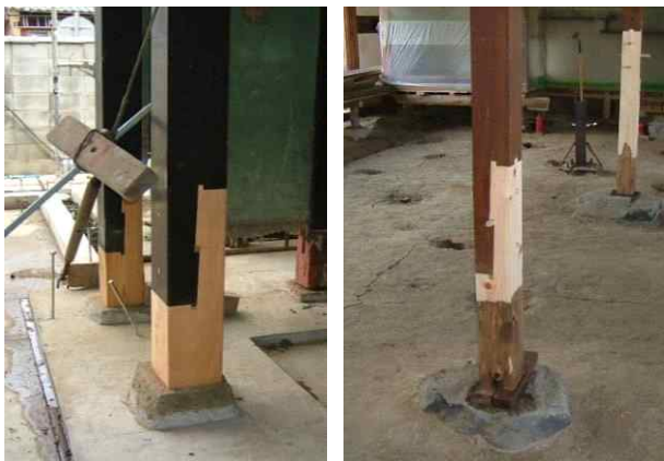
Fig.4 Repair of Wooden Member Damaged by Termites
