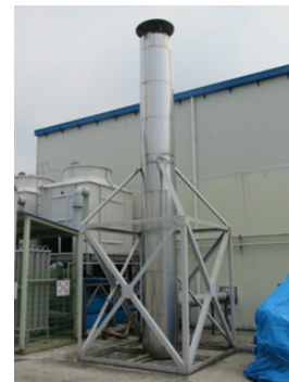
Fig. 7 Micro gas turbine exhaust duct
