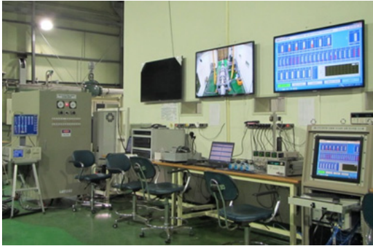
Fig. 8 Micro gas turbine control and monitoring room
