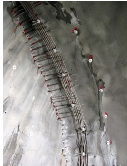
Fig. 5. Principle for excavation through poor stability weakness zones based on short round lengths, spiling and reinforced ribs of sprayed concrete (top; based on NFF, 2008), and photo illustrating spiling and shotcrete ribs in tunnel with heavy support also of the face (right)
