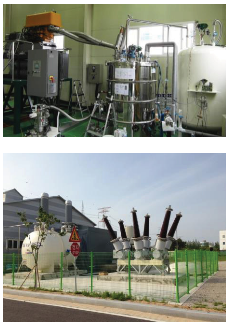
Fig. 3. The cooling system constructed at the site
