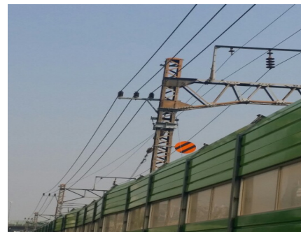
Fig. 13 Railway 22.9kV Aerial Transm -ission lines
