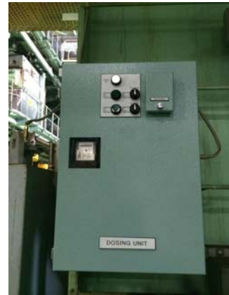
Figure 6: Dosing unit including dosing pump
