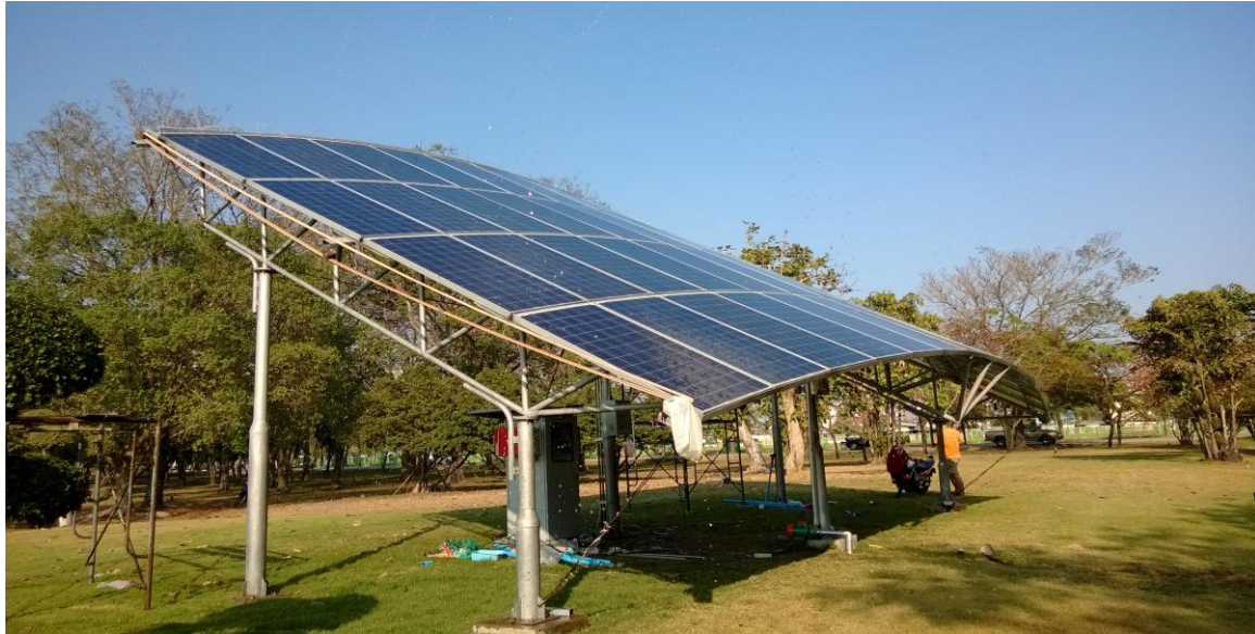
Figure 7. Other side of 10kWp photovoltaic system.
