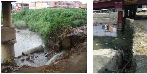
Fig. 6 Change in river bank under Chabhail Ringroad Bridge. (2005 and 2014)
