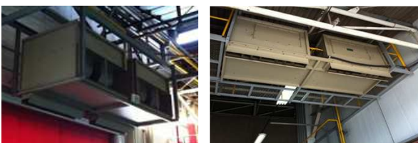
Fig. 1 Air-curtain in a large-scale factory and installed distance at the opening
