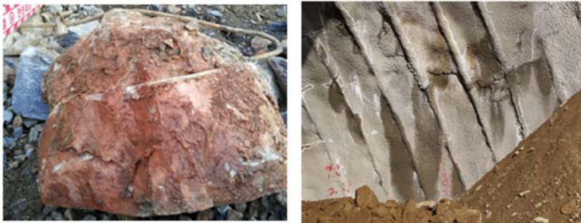
Fig. 6. Damaged rock bolt and clay seam in discontinuities (left), and tension cracking of shotcrete on the side wall of the No. 2 tunnel.
