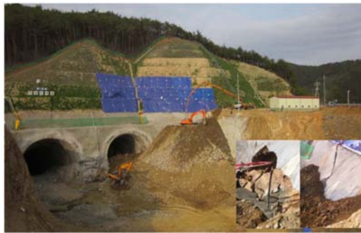
Fig. 17. Cavity concrete filling and counterweight fill construction (4 days after the slope failure).
