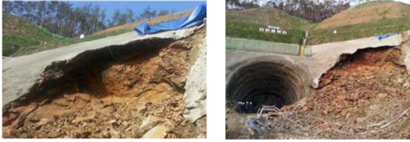
Fig. 4. Failed rock mass. Note the scale of the failed rock mass compared with the tunnel diameter of 12.8 m.
