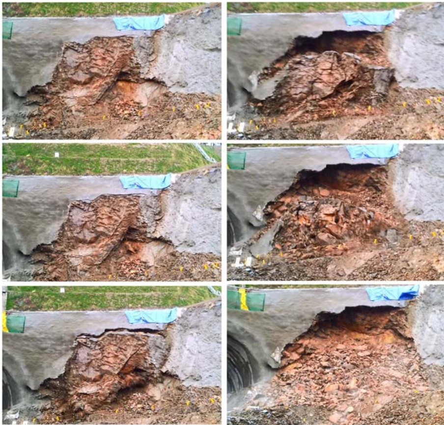
Fig. 3. Time-lapse photographs of the rock-slope failure.
