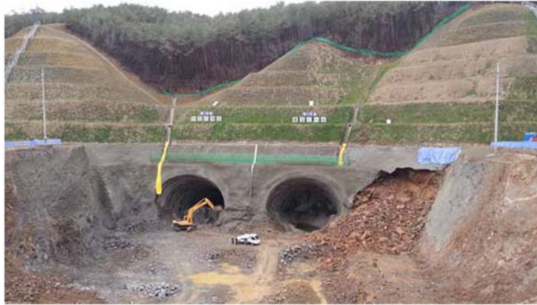
Fig. 2. Slope failure of a large-scale cut slope at a tunnel portal.
