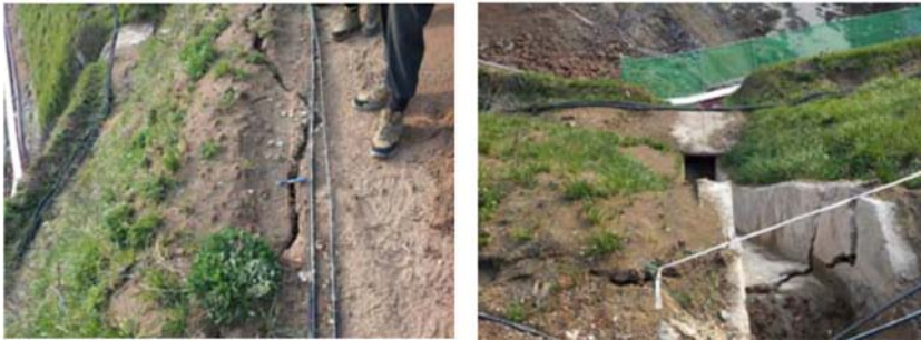
Fig. 5. Longitudinal tension crack developed along the berm above the failure slope.
