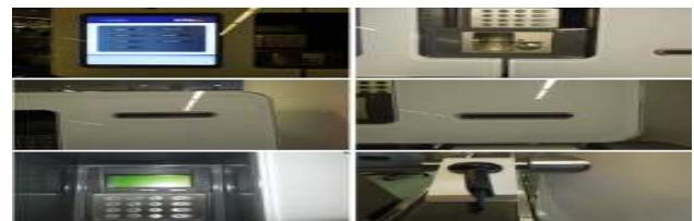
Fig. 9 Composition of SBD Equipment and systems of Brussels Airport
