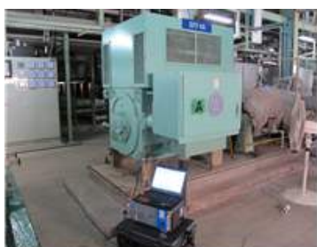
(b) on-line PD testing system
