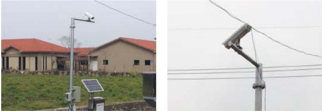
Fig. 3. CCTV system for outflow of the image acquisition at Seong-eup bridge.
