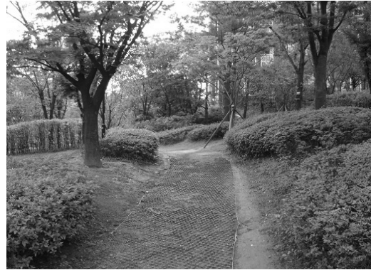
Permeable pavement (Suwon Woncheon 1 park)
