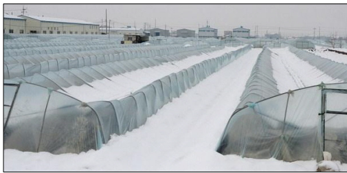
[Fig. 1] Greenhouse Collapse by Snow Load
