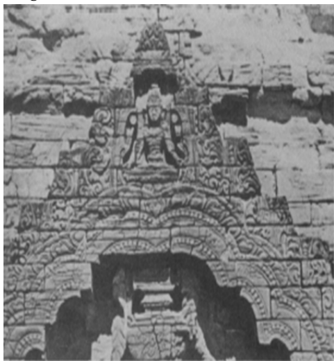
Location: on the top of the perforated stone window at Nanpaya Temple
