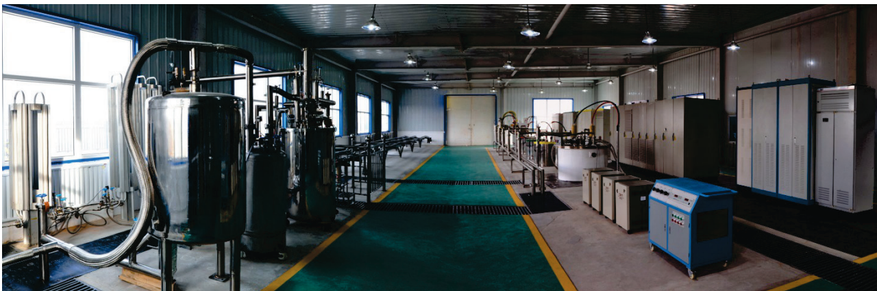
Fig. 3. 10kV superconducting power substation at Baiyin Industrial Park [3].
