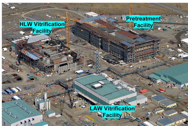
Fig. 1. Aerial photograph of the WTP under construction at DOE's Hanford Site in Washington State (as of July 2014, Source: www.hanfordvitplant.com).
