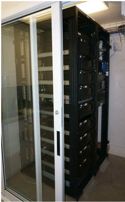
Figure 5. CCD Control computers, PC-TCS & AUX Computer are installed in the KMTNet Observatory at CTIO.
