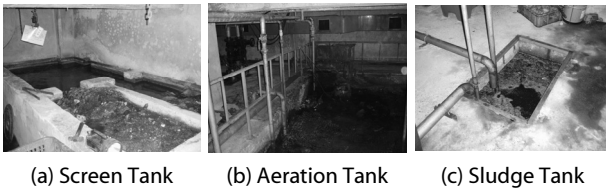
Fig. 4. Existing Wastewater Treatment Facilities
