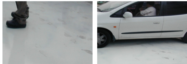
Photo 2. "Tacky" phenomenon on the waterproofing layer
