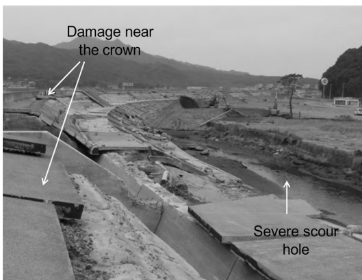
(a) Damaged sea-dike
