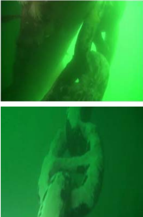
Fig. 18 Underwater inspection of mooring chains (upper: contact part of chain guide, lower: center part of mooring chain catenary)
