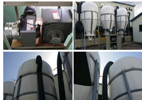
Fig. 3. Feed Bin ventilation system
