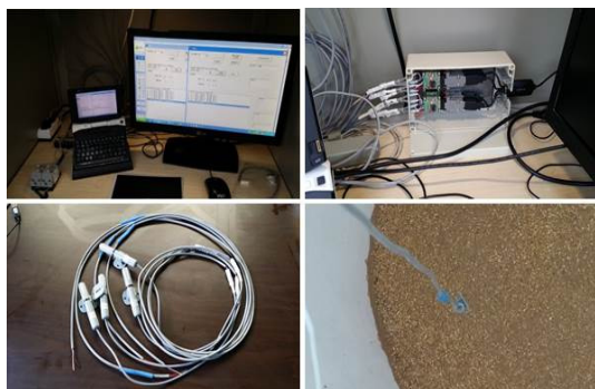
Fig. 2. Temperature/humidity sensor and data server
