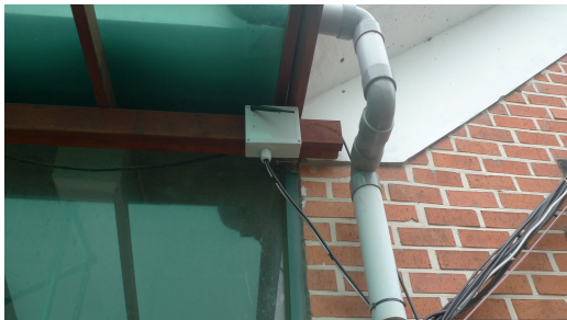
(b) Installed location of receiver
