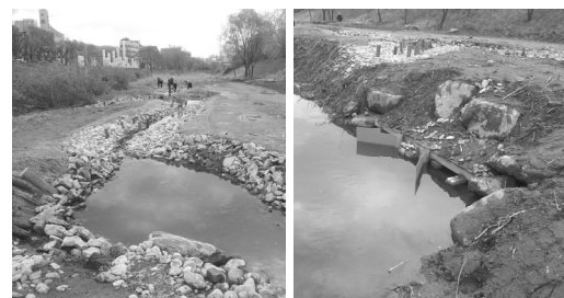
Figure 8. Gravel bed channel & enlargement of outlet in wetland. Photo from Eco Innovation, 2013.
