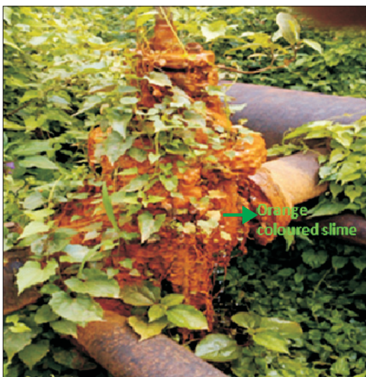
Fig. 1. Macroscopic orange coloured (acidic) slime formation in a leaking valve of water flow line in Source Well Manifold.
