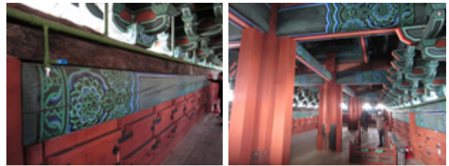
(b) Deflection of main horizontal beams on 2 nd floor
