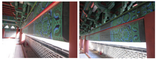
(a) Deflection of main horizontal beams on 1 st floor
