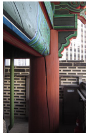
(c) Column splitting on 1 st floor
